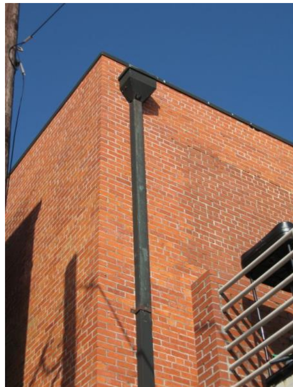
A downspout like this at 614 Main Street should be kept in good repair.
