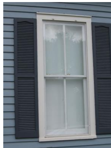
The storm windows at 508 Ibert Street are appropriate models.
