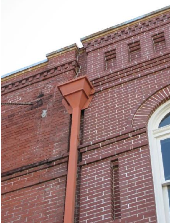
Downspouts, like this at 608 Main Street, help protect buildings from water damage.
