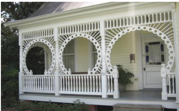
The detailed porch at 211 Clark Street required careful painting for proper maintenance.
