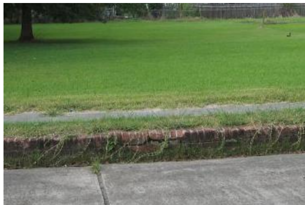
Other site elements, like this brick wall in the 700 block of 1st Street, should be preserved and maintained.
