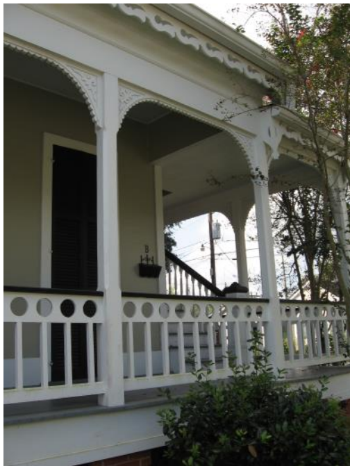
If wood elements like the porch trim on this house at 309 Adams Street is maintained, it can last indefinitely.
