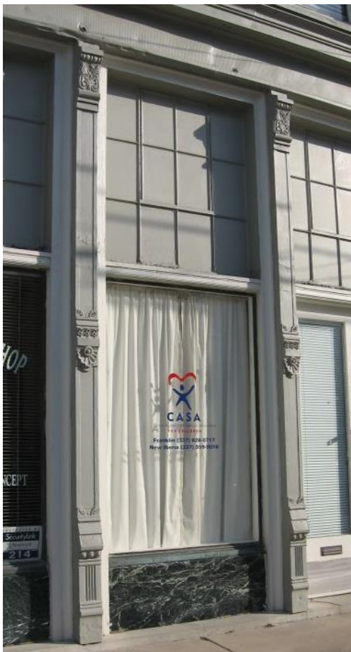
The painted finish of these cast iron columns at 212 Willow Street helps to protect them.
