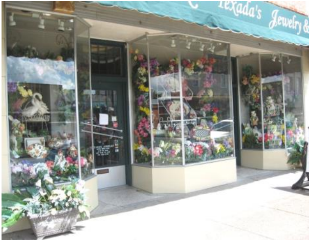
Large display windows and bulkheads beneath them, like these at 606 Main Street, are traditional storefront elements. These bulkheads have applied Carrara glass
