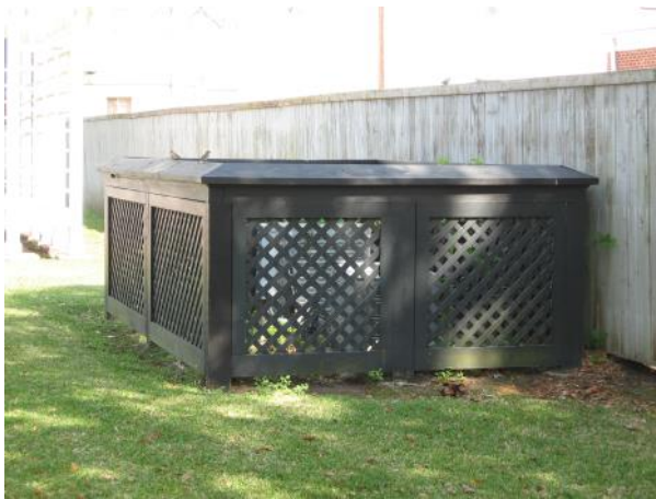
An attractive wood lattice screening of a HVAC unit at 808 1st Street
