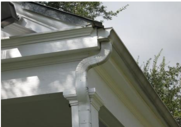
The downspout on 301 Iberia Street uses placement at a corner and coloring that matches its adjoining surface to minimize its visual effect.
