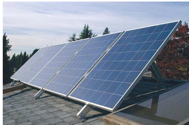
Solar panels should only be added at rear elevations or rooflines not readily visible from the street.
