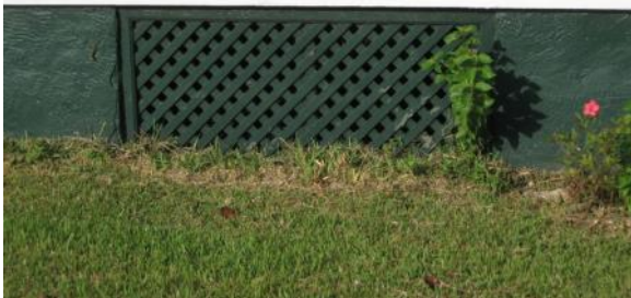
The pier foundation at 817 Main Street has appropriately been left visible, with lattice inserted in between piers, rather than covering them.
