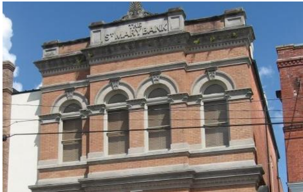
Upper windows, like these at 614 Main Street, are defining elements of upper facades.
