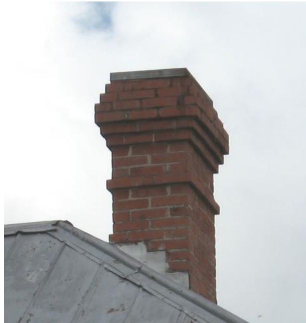
The distinctive corbelled brick chimney at 600 Adams Street should be reconstructed to match its historic appearance if it needs extensive repairs or replacement.
