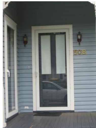
Storm doors should be full-view, so that the main door is visible (508 Ibert Street).
