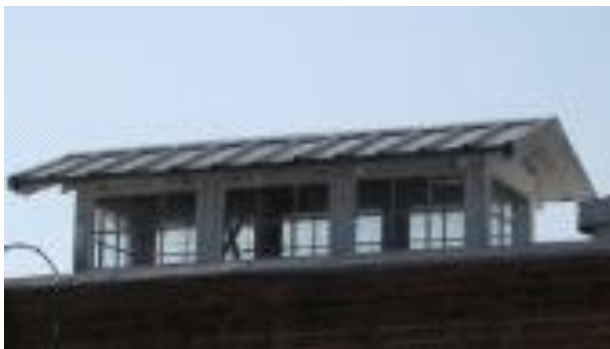
This original skylight monitor at 726 Main Street is a unique roof feature that should be preserved.
