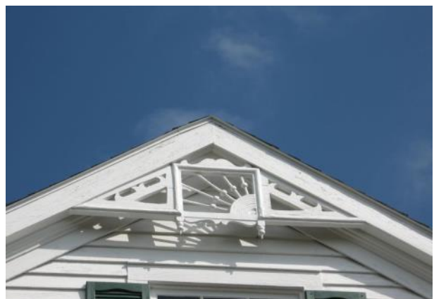
The paint on this historic vergeboard at 800 2nd Street maintains historic character and helps with physical preservation.
