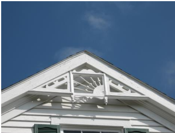
Detailing such as this sunburst design in the gable field at 800 2nd Street should never be removed or concealed.
