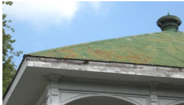
The metal roofing materials at 216 Commercial Street contribute to the house's historic character.
