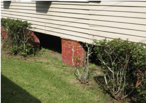
The brick pier foundation of the house at 807 2nd Street has been appropriately left uncovered.
