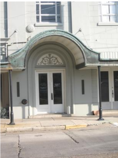
This copper and wood canopy at 200 Willow Street is significant in defining this entrance and should be preserved and maintained.
